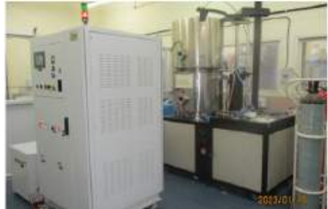
Figure A.4.24: Pulsed HV DC power supply integrated with plasma nitriding system at IGCAR, Kalpakkam.
