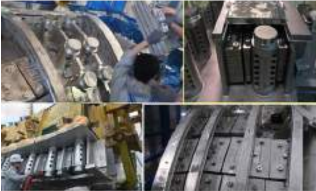
Figure B.1.4: In sequence : IWS lowered for assembly in VV sector; IWS assemble around flexible support housing between outer and inner shells of VV, inspection after assembly to ascertain needed clearance, VV segment view after assembly of IWS and ready for welding the outer shell.
