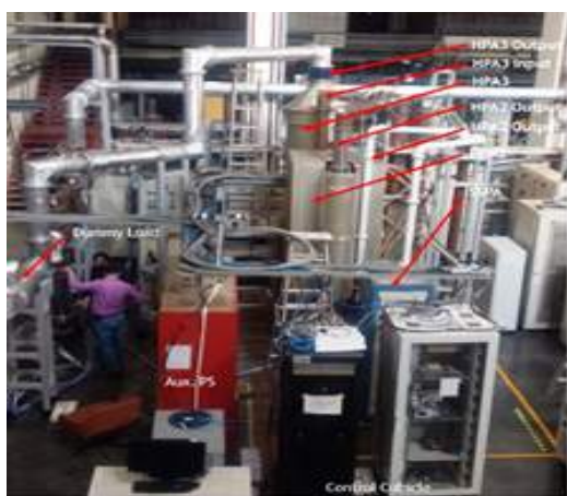
Figure A.3.10: View of Installed RF source in SST-1 hall.
