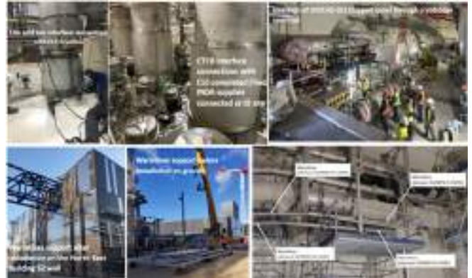
Figure B.1.5: Installation of X, Y cryolines and warmlines at ITER site.
