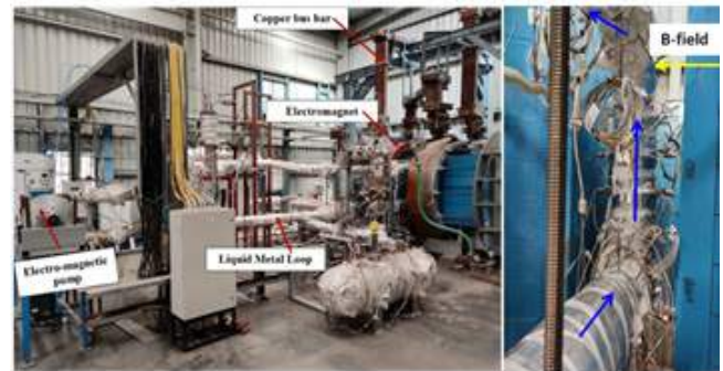
Figure A.4.6: Pb-Li MHD loop at the institute (left) and 'U' shaped circular cross-section test mock up inside the magnet pole gap (right).
