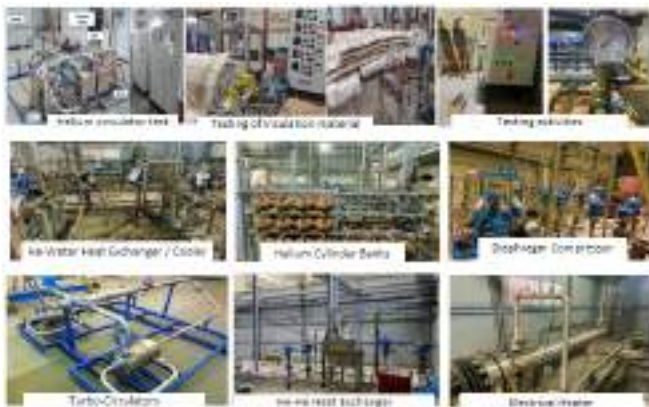
Figure A.4.5: Major components of the EHCL system installed, integrated and tested at site.
