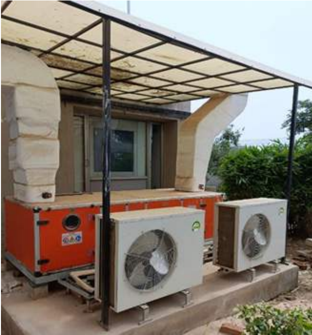
Figure D.2: Direct expansion air handling unit and air conditioning system is for existing class 10000 clean room for SRP Lab at FCIPT campus.
