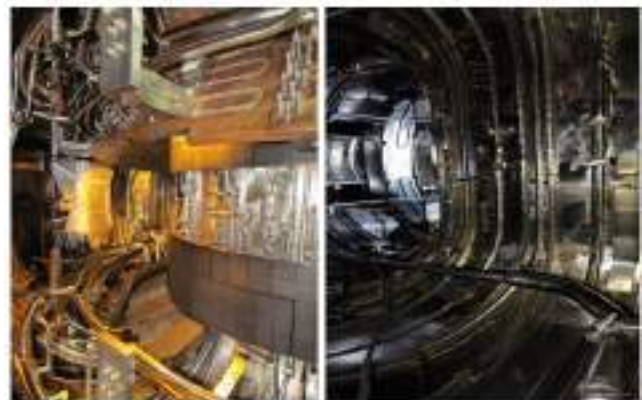
Figure A.3.8: Inside view of SST-1 vacuum vessel before and after PFCs removal.
